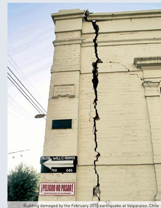
Building damaged by the February 2010 earthquake at Valparaíso, Chile
