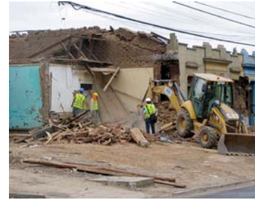
Figure 6. Collapse and demolition of adobe brick structures in Talca (Source: AIR)
