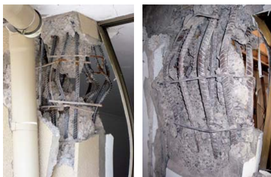
Figure 10. Large buckling of the vertical reinforcement bars exacerbated by the lack of enough lateral, or confinement reinforcement (Source: AIR)
