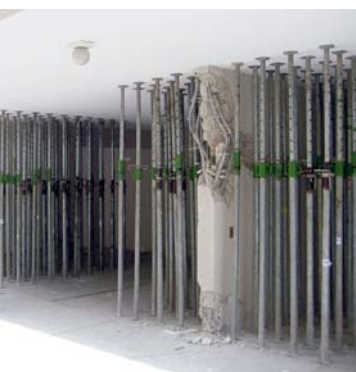
Figure 9. Partial collapse of shear walls (Source: AIR)
