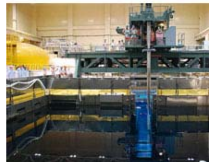
Figure 7. Spent fuel storage pools (top) showing fuel assembly being moved through gate between pool and reactor top. Yellow object is removed core dome. Steam emanating from the fuel storage pool in unit 4 on March 15, 2011, under the loading crane showing at the center of the picture (bottom).
