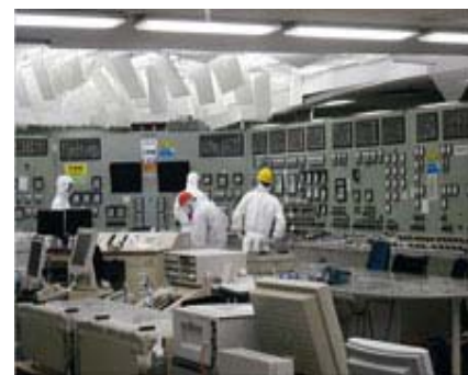
Figure 1. Station Blackout loss of power to the control room of the Fukushima Daiichi unit 1 reactor on March 24, 2011 (left). Restoring offsite power to units 1 and 2 and power to the control room of unit 2 on March 26, 2011
